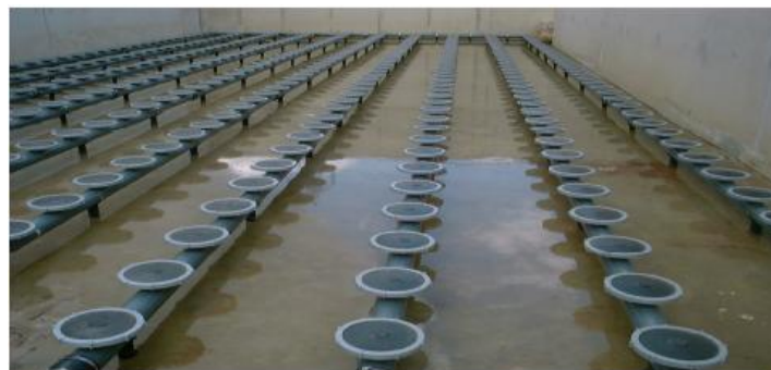
Figure 5.6: Fine bubble disc diffused aeration system (126)
