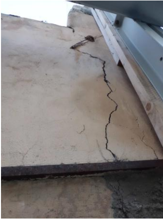
Figure 3.119 Tie Rod Crack
