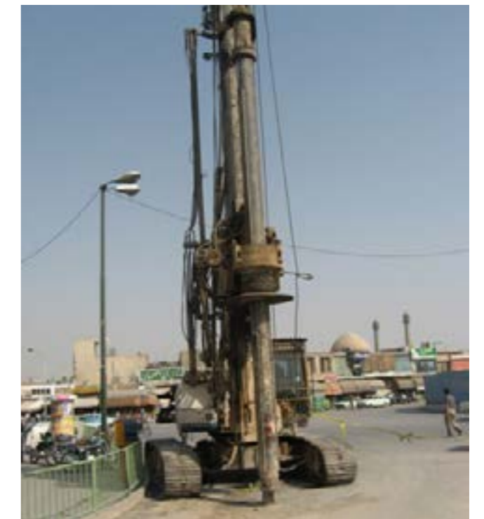
102 .excavation in proximity of the heritage mosque; heavy drilling machine trembles the old area and the heritage (source: NAQSH, E, JAHAN-PARS Consulting Engineers, 2010.)
