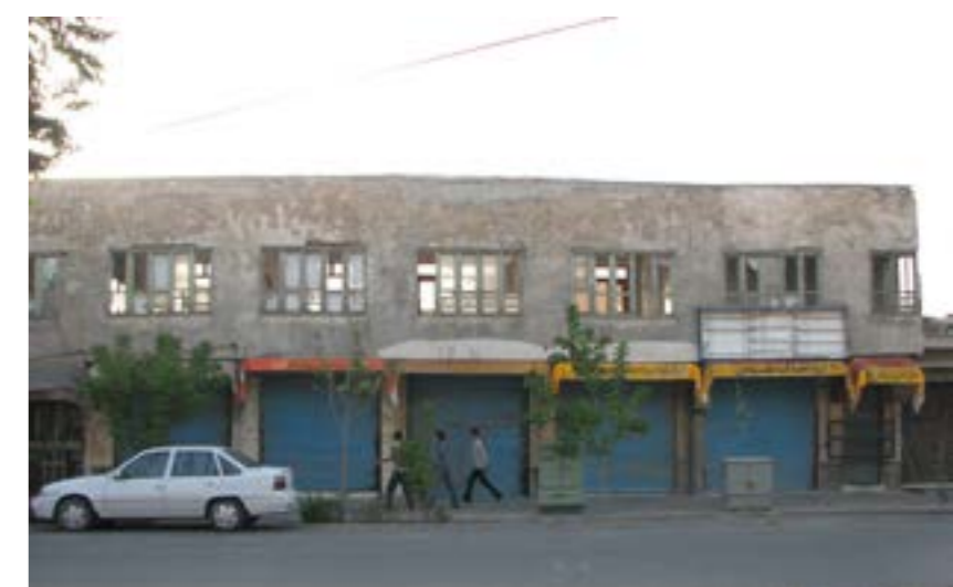
125.broken windows, dismissed plot in the area. (source: NAQSH, E, JAHAN-PARS) Consulting Engineers, 2010.)
