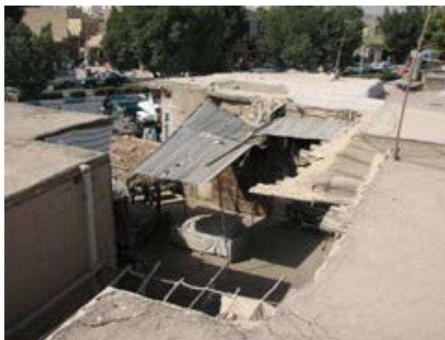
86.blighted and degraded active plots in the area (source: http://www.panoramio.com )
