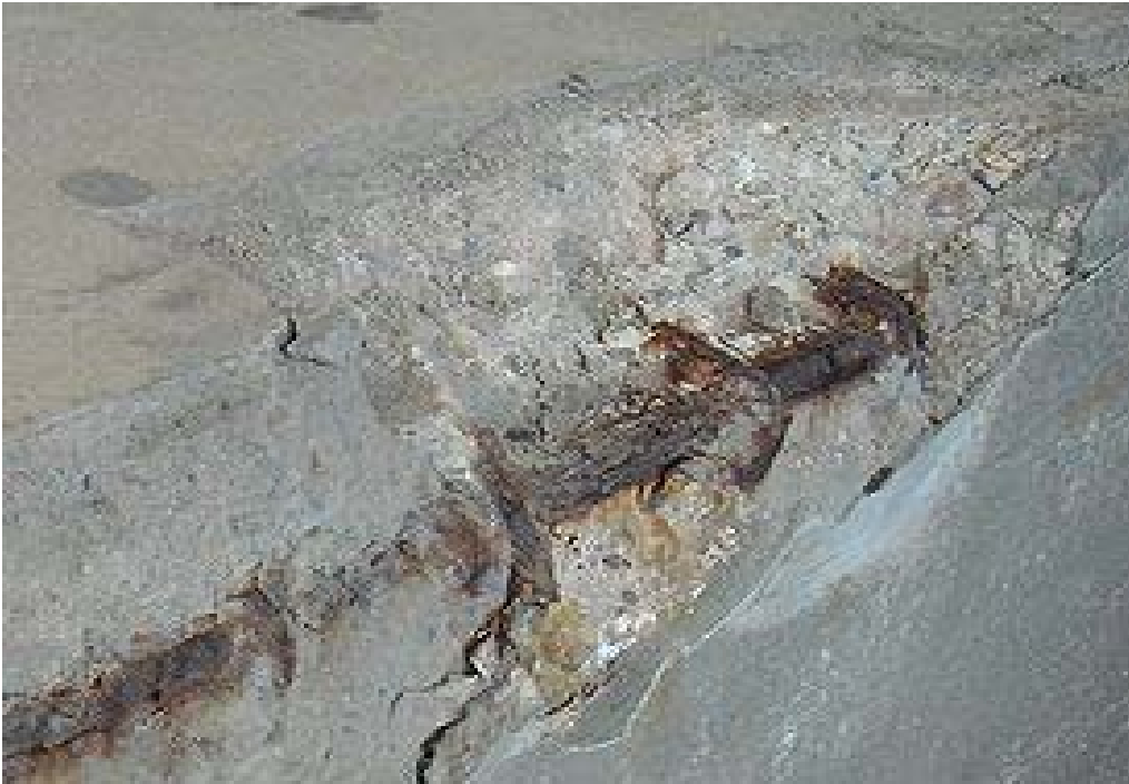
Figure 2. 7: Example of degradation in concrete
