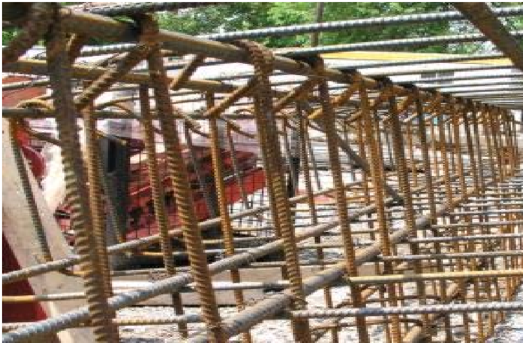
Figure 2.1: A tied rebar beam cage. This will be embedded inside cast concrete to increase the tensile strength of the concrete.
