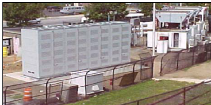
Figure 1.6. NewYork Electric Power 1.2MW / 7.2MWh Sodium Sulfur Battery Facility [3].
