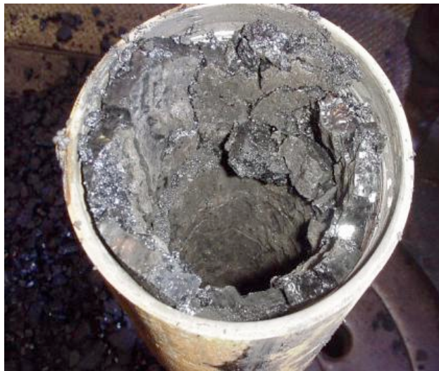
Fig.32: Asphaltene deposited layer on the internal wall of a pipeline.
