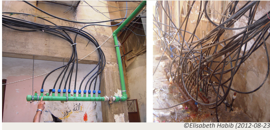
Photo 4-10: The EU funded project (on the right) replaced the old rusted water supply system (on the left) and elevated it in order to increase the pressure of the water and to ensure the efficiency of the whole network
