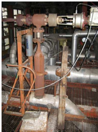
Figure 2.5 Pneumatic actuator of loop pressure control valve (V4).
