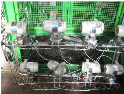
Figure 2.7 Differential pressure transducers installed along channel A.
