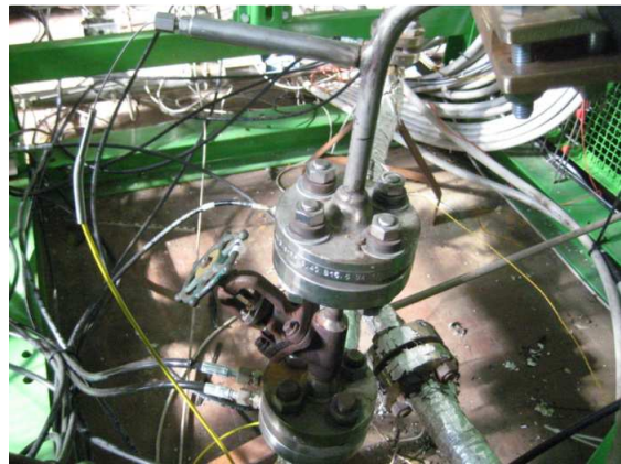
Figure 2.6 Calibrated orifice and channel inlet valve.
