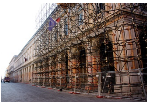
FIG. 6.17: CITY CENTRE OF L’AQUILA: 4 YEARS AFTER THE EARTHQUAKE
