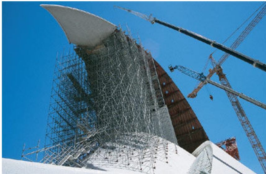
Figure 31 - Modular scaffolding served as shoring for the construction of the winged-shaped roof. Anchoring was carried out using a 1.50 x 1.50 m square grid formation on the “nut” roof shell. Base spindles were used to vertically adjust the prop lengths for the different contact area levels
