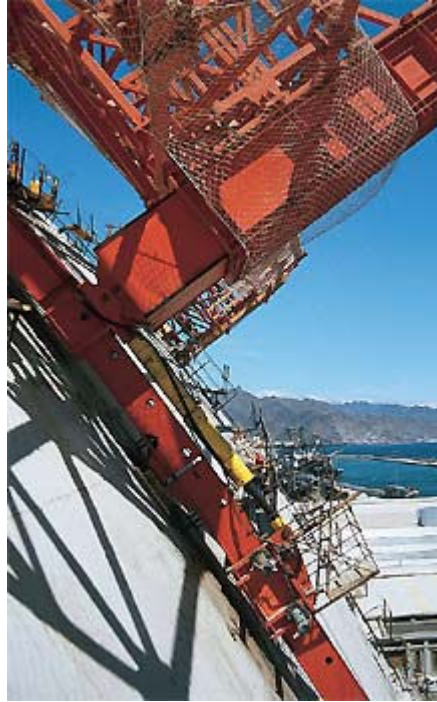
Figure 30 - One of the two climbing units which hydraulically lifted the complete construction, including working platforms and formwork, from cycle to cycle
