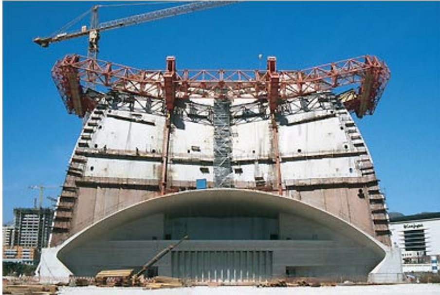
Figure 32 - All carriage movements are carried out using three independently operated hydraulic circuits: moving forward and retracting, positioning as well as shuttering and striking.
