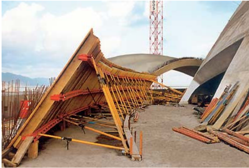
Figure 25 - Positioning of the internal formwork for the curved and inclining sail-like walls, anchoring the supports in the suspended intermediate slab served to carry the high horizontal loads from the bracing
