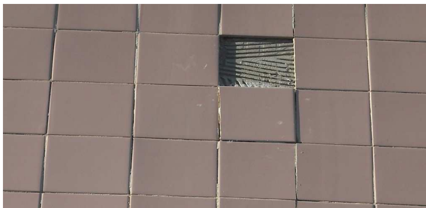
Figure 3.7 - Detachment detail of the excluded façade
