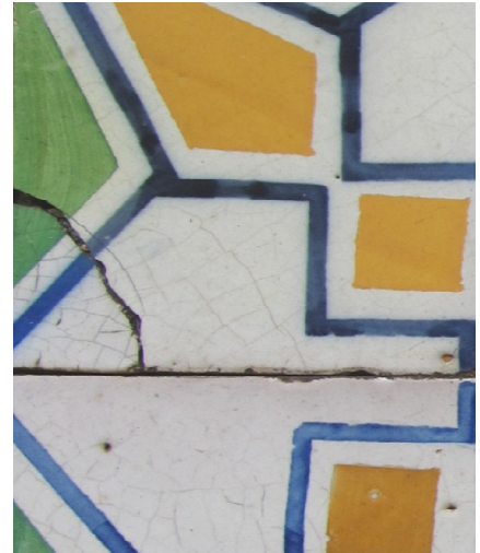
Cracking without predominant direction
