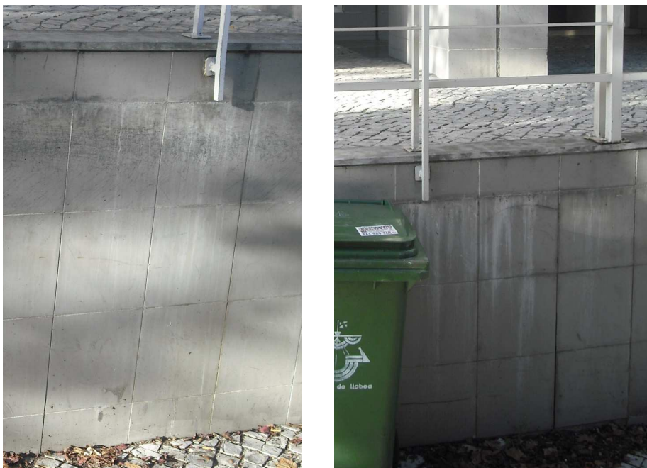
Figure 3.8 - Evidence of the anomalous state of deterioration of the excluded building
