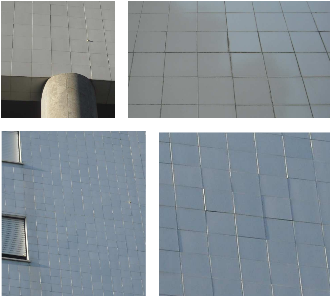
Figure 3.9 - Lack of flatness of the cladding in the building located in Rua José Escada.
