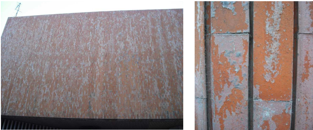
Figure 3.4 - Façade excluded; on the right a detail of the efflorescence affecting the cladding
