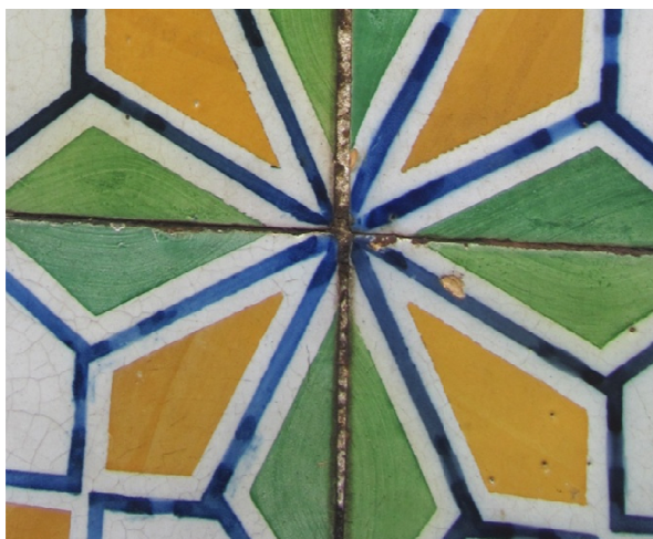
Joint deterioration without loss of material
