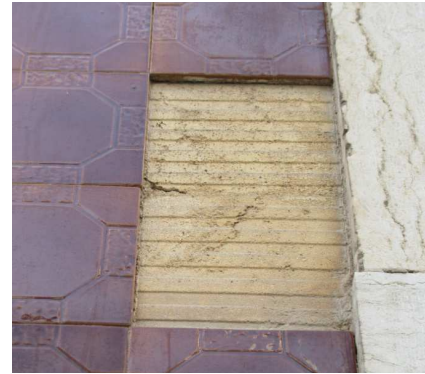
Figure 3.43 - Excluded façade: the mortar has not been adequately pressed
