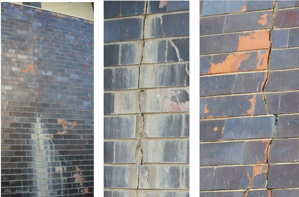
Figure 3.5 - Cracking in the building in Avenida do Infante Santo.
