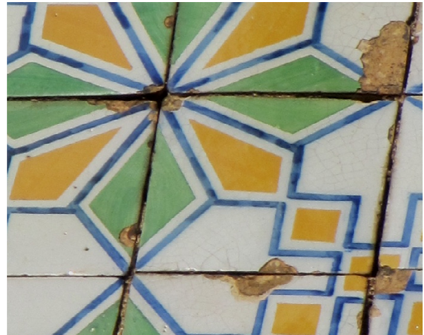
Joint deterioration with loss of material
