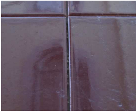
Figure 3.42 - Façade featuring joints deterioration
