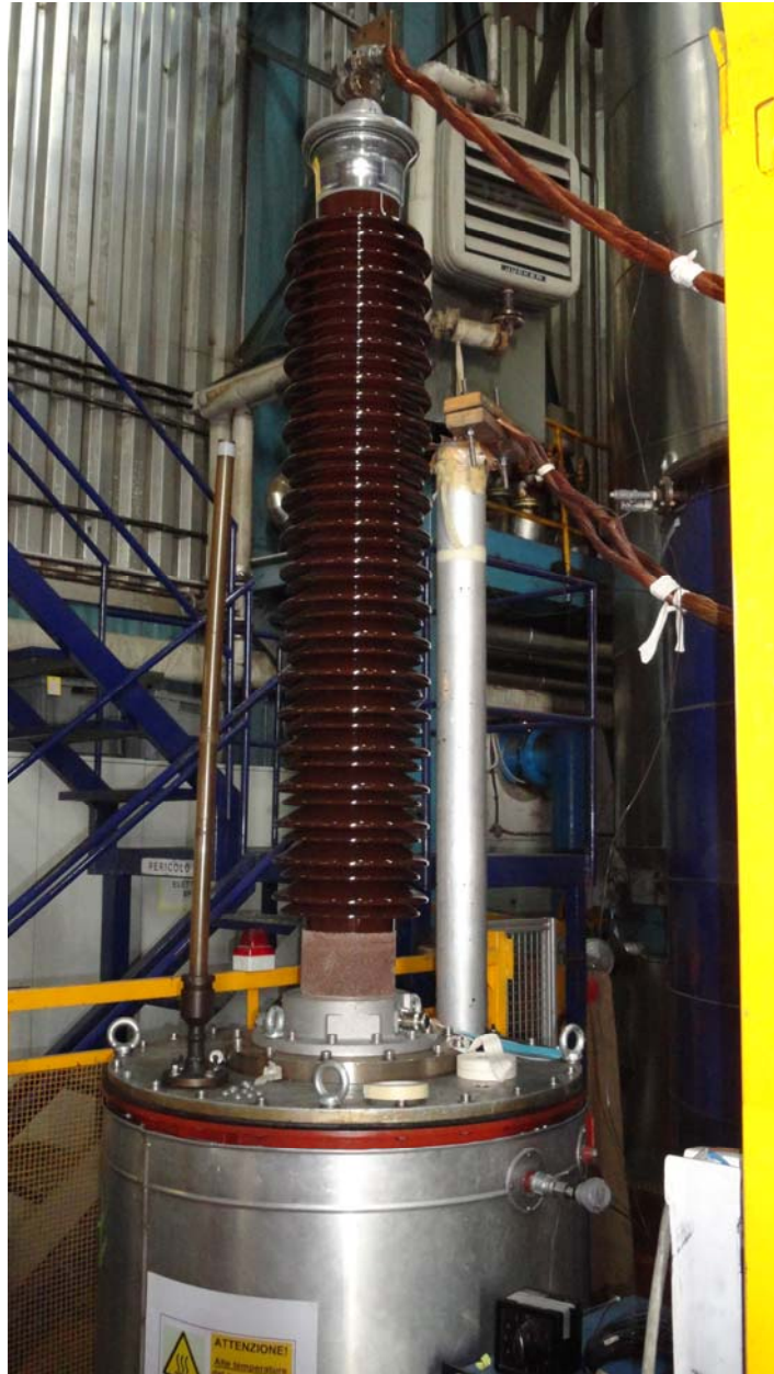
Figure 2.4 - A Draw Lead Bushing Mounted on an Oil Tank During The Temperature Rise Test
