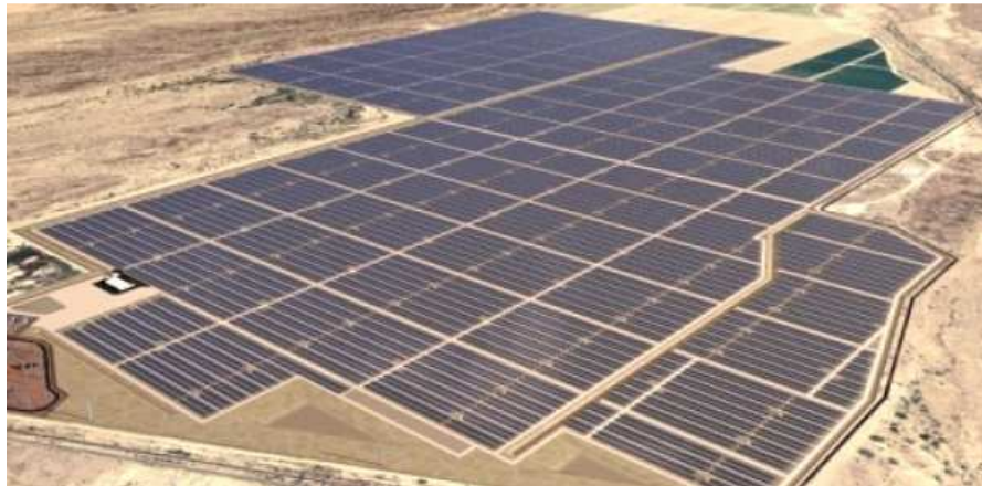
Figure 1-5: Agua Caliente PV facility
