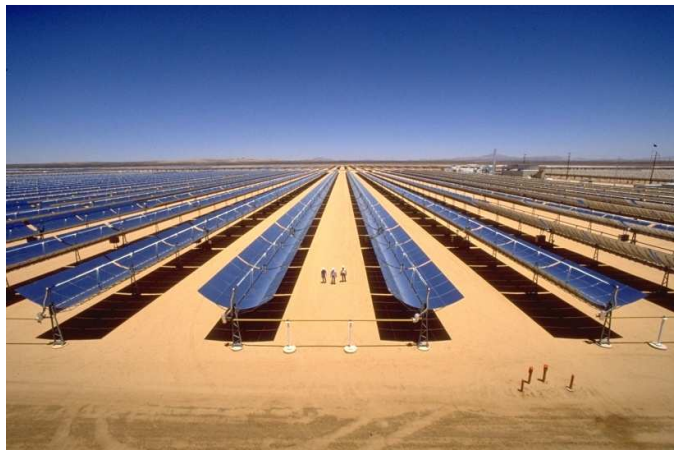
Figure 1-10: Parabolic trough solar field
