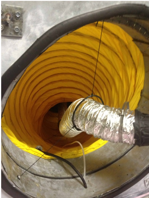
Figure 5.6. The silver duct's hanger
