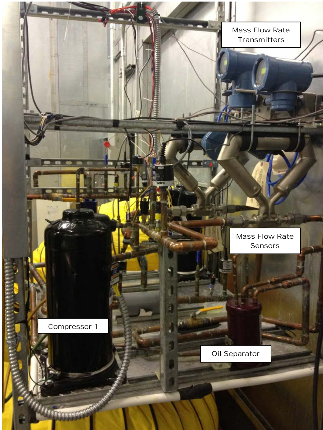
Figure 3.28. The new piping and sensors of the experimental set-up.
