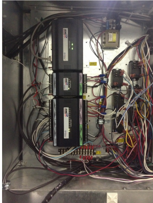
Figure 3.31. The new controller and wiring (magnification of fig.3.29).
