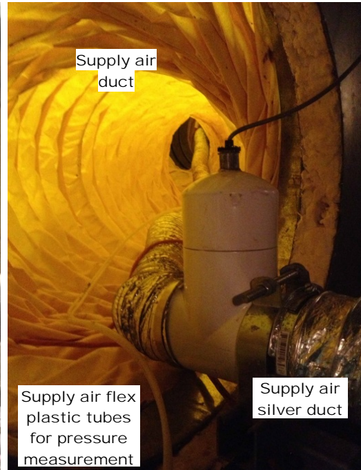
Figure 5.7. View of the yellow duct from the inside.
