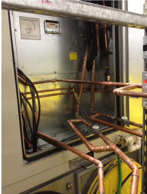
Figure 3.30. Connections from the existing piping to the new apparatus.
