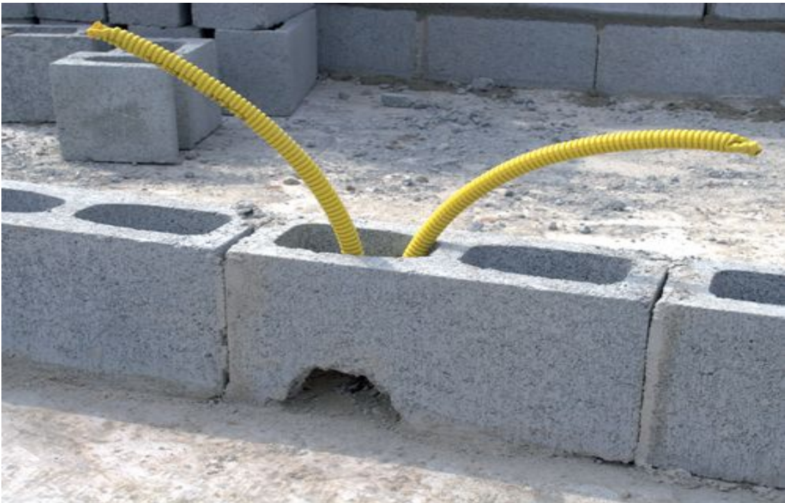
Figure 25: Electric ducts passing through precast concrete blocks roles
