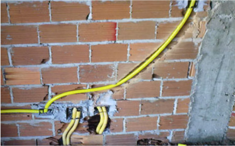
Figure 24: Tears in the wall for placing electric ducts
