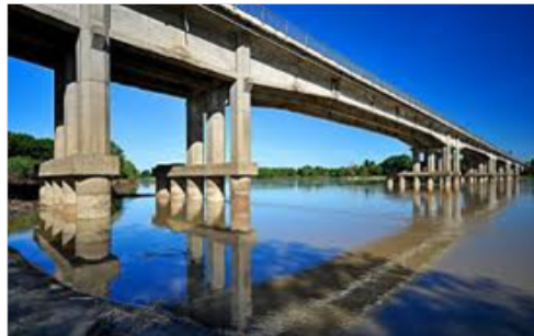
(a) Undermined bridge.
