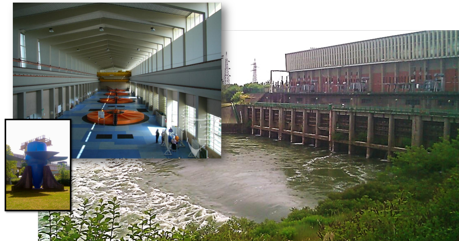
Figure 5.4: Outside and inside view of IS power station with its four Kaplan turbines
