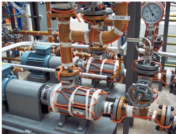
Figure 3.36- Heating equipment system
