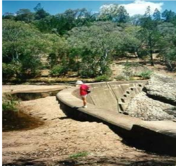
Fig. 1. 4: Functional failure of Dam due to sedimentation.
