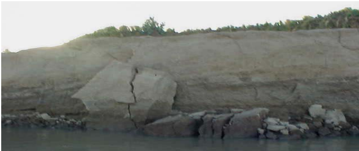
Fig 7. 9: Bank erosion in the main Nile.
