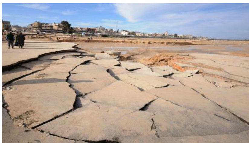
Fig. 1. 5 : Roads collapse in Sinai-Egypt due to erosion and sediment transport.
