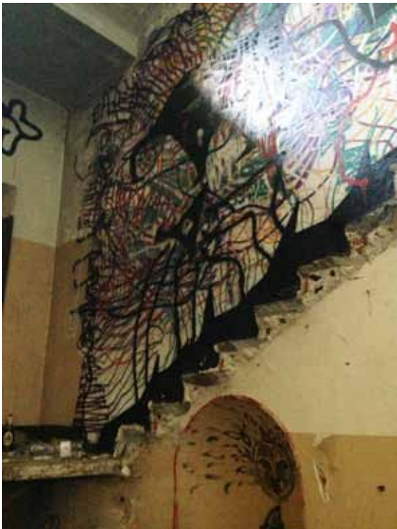
12 - Original destroyed stair
