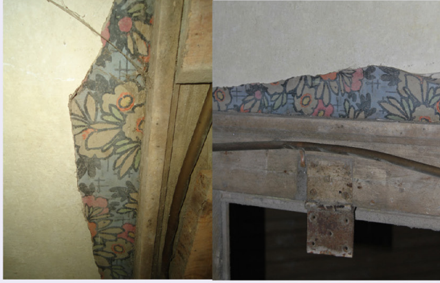
View from the two remaining pieces of the wallpaper left in the house.
