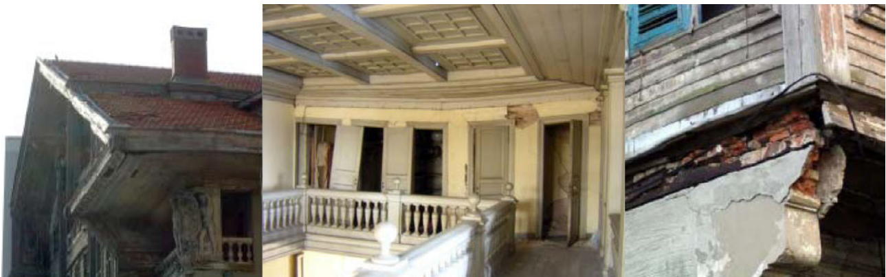
Figure 55: a) View from a Box gutter that divides the North slope into upper and lower halves. b) Picture of the deflection of the frame. c) Decay of the Iron protection.
