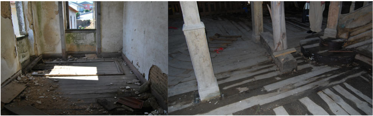
Figure 41: View of the Typical Pavements on the Services Room and on the main Hall.
