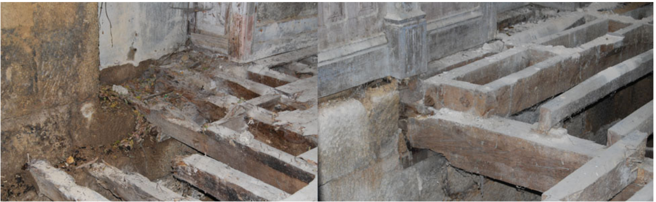
Figure 22: Detailed Pictures of the connection between the bearing wall and the wood structure of the floor
