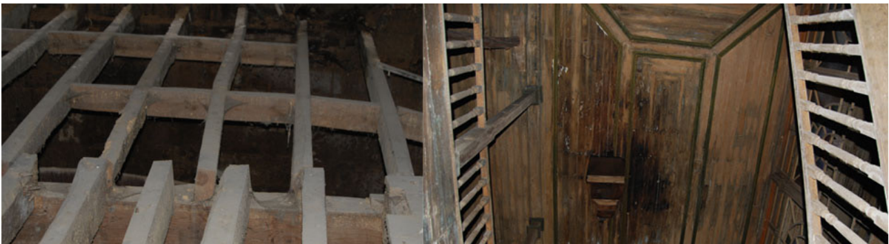
Figure 25: View from the structure on the Ground Floor. View from the second-floor ceiling.
