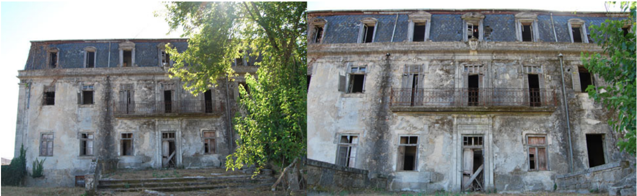
Figure 37: View of the South-East Façade. Coser view of the central structure of the façade.
