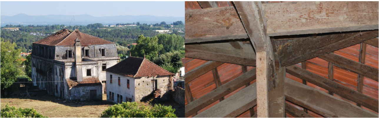
Figure 23: View of the Main Roof. Detail of the roof structure on the Annex Services Building.
