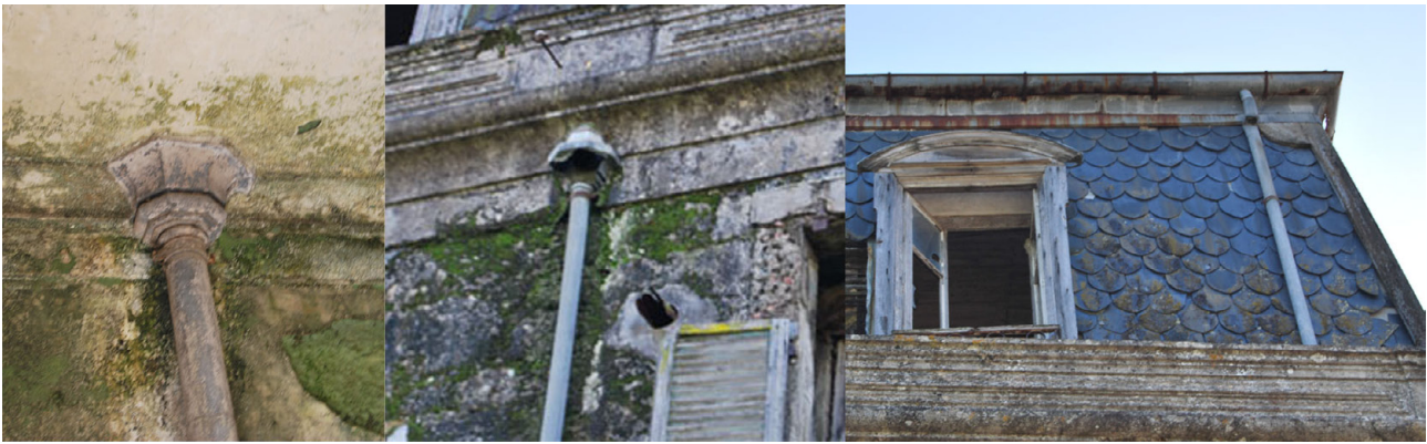
Figure 32: View from a bathroom pipe inside the house. View from the external drainage system on the Garden Façade. View from the Gutters on the North-West Façade.
