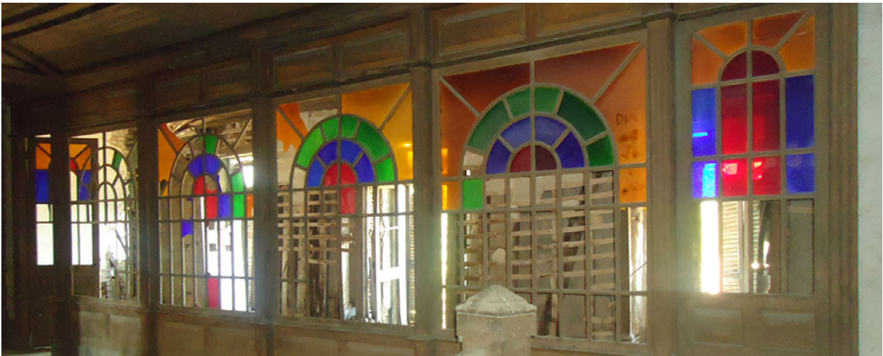
Figure 34: View from the wood panel behind the main stairs decorated with coloured glass.
