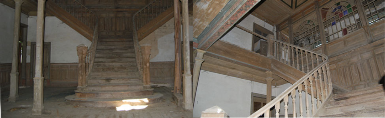
Figure 43: Main Stair's Picture. Secondary Stairs of the Kitchen and Access to the second Floor respectively.
