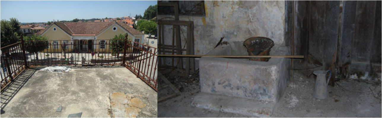
Figure 30: Cement of the floor of the front balcony. View of the floor of the kitchen.
