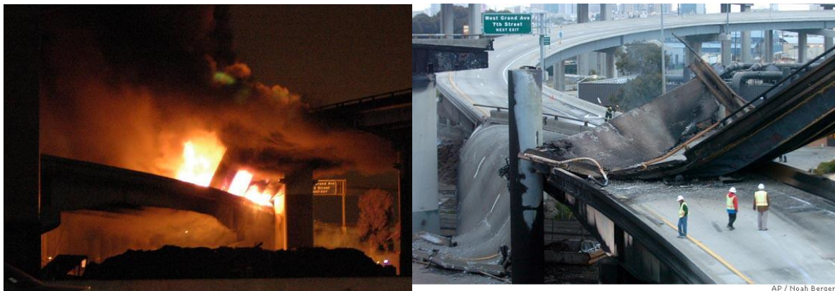
Figure 1.7: McArthur Maze Collapse by Fire (L. Giuliani et al.).
