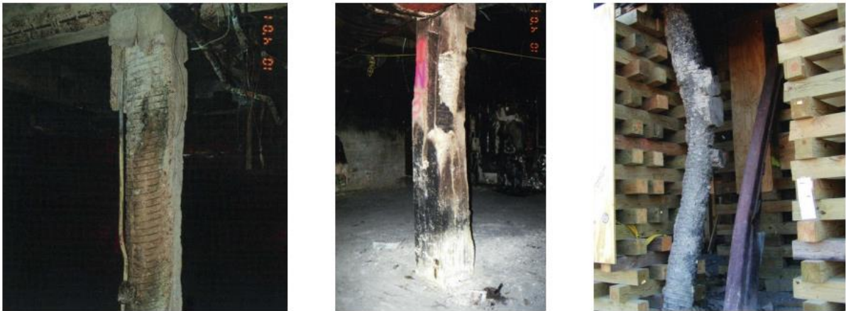
Figure 1.2: Seriously damaged due to spalling of columns (Explosive spalling).
