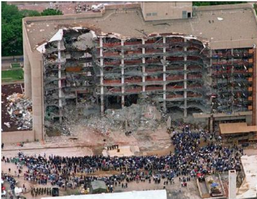
Figura 2.1.2 Alfred P. Murrah Federal Building, Oklahoma (1995)
