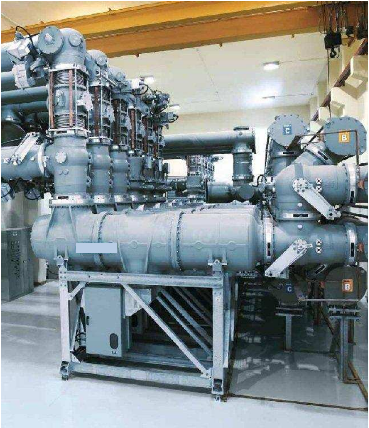
Figure 2.3 - 420 kV GIS circuit-breaker in a Gas Insulated Electrical Station
