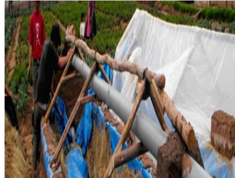
Figura 4.57 Shed - roof digester.
