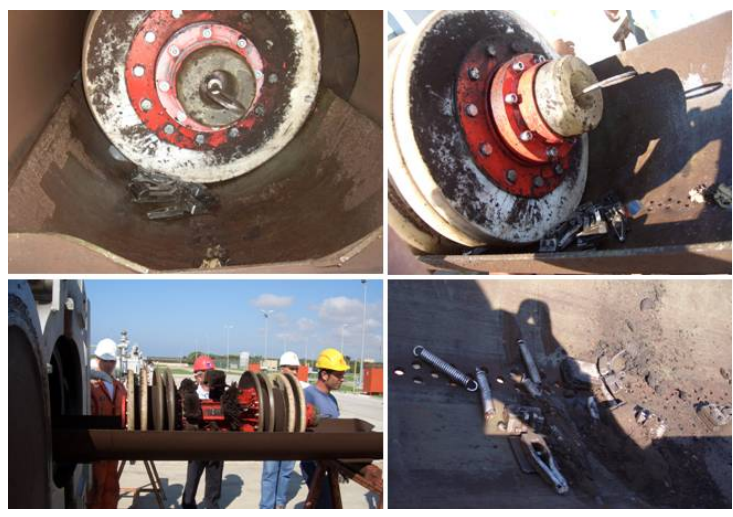
Figure 6.12: PIG2 arrival, carrying fragments of previous damaged PIG1.
