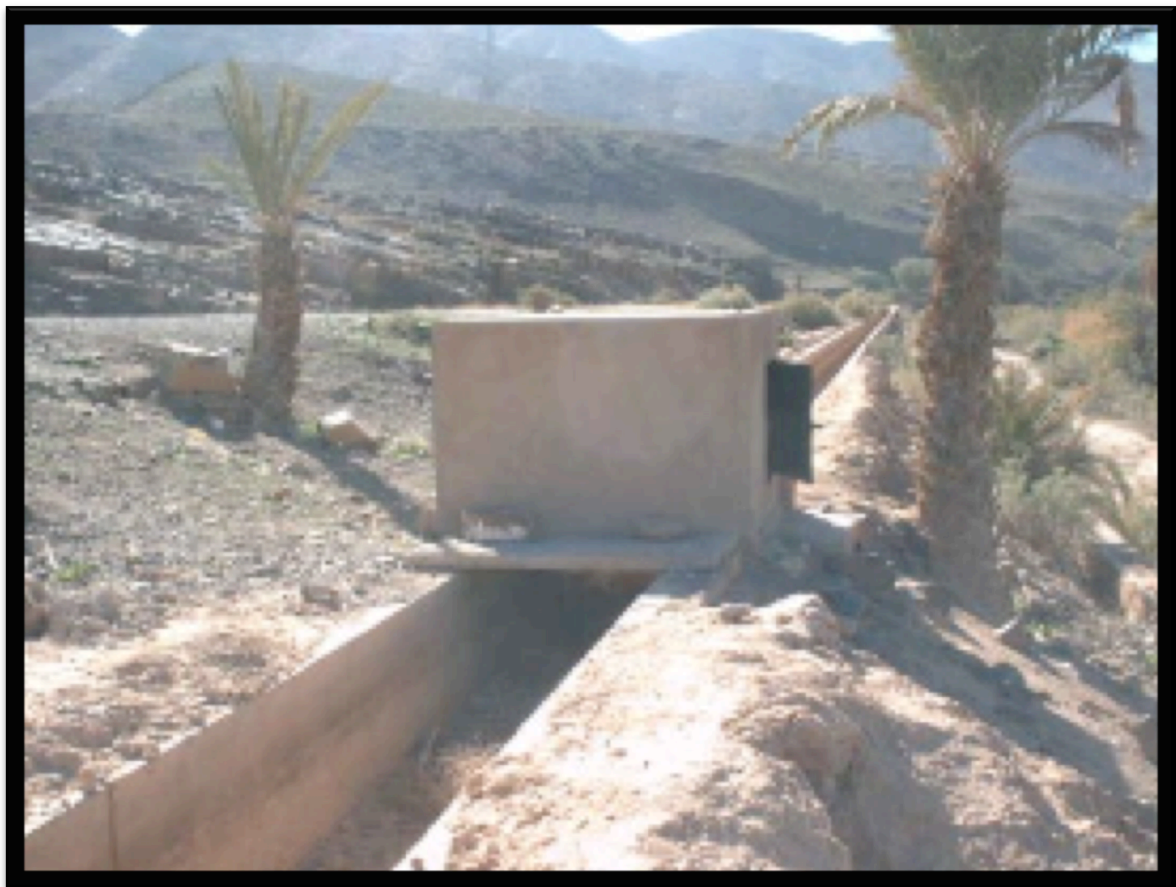
Figure 26: one of the distribution water channels (at the bottom)
