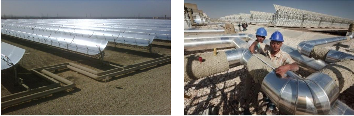
Figure 3.4 Extra lengths needed for thermal expansion (left). Posing of pipe insulation (right) (Kuraymat-Egypt) [14]
