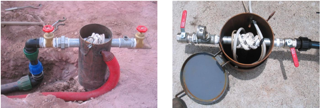
Figure 3.4 Side view and top view of the well with the underwater pumping system installed
