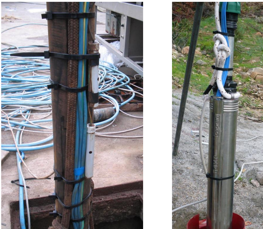
Figure 3.16 Standard tie mechanism used in the underwater pumping systems
