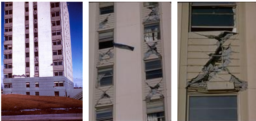
Figure 2.3 – Failure of coupling beams due to earthquake Alaska (Alaska Digital Archive)
