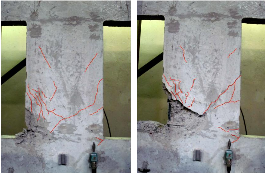
Figure 6.12 – Coupling beams with both longitudinal and transverse reinforcement under increased cyclic displacements
