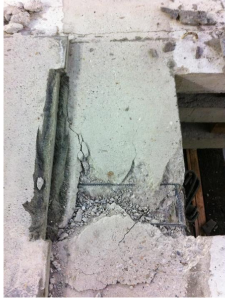
Figure 6.23 – Coupling beam strengthened with HPCRCC under cyclic loading – manual remove of the HPCRCC layer at the end of test
