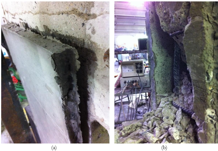
Figure 6.22 – Coupling beam strengthened with HPFRCC under cyclic loading: (a) delamination and (b) buckling of bars under negative loading
