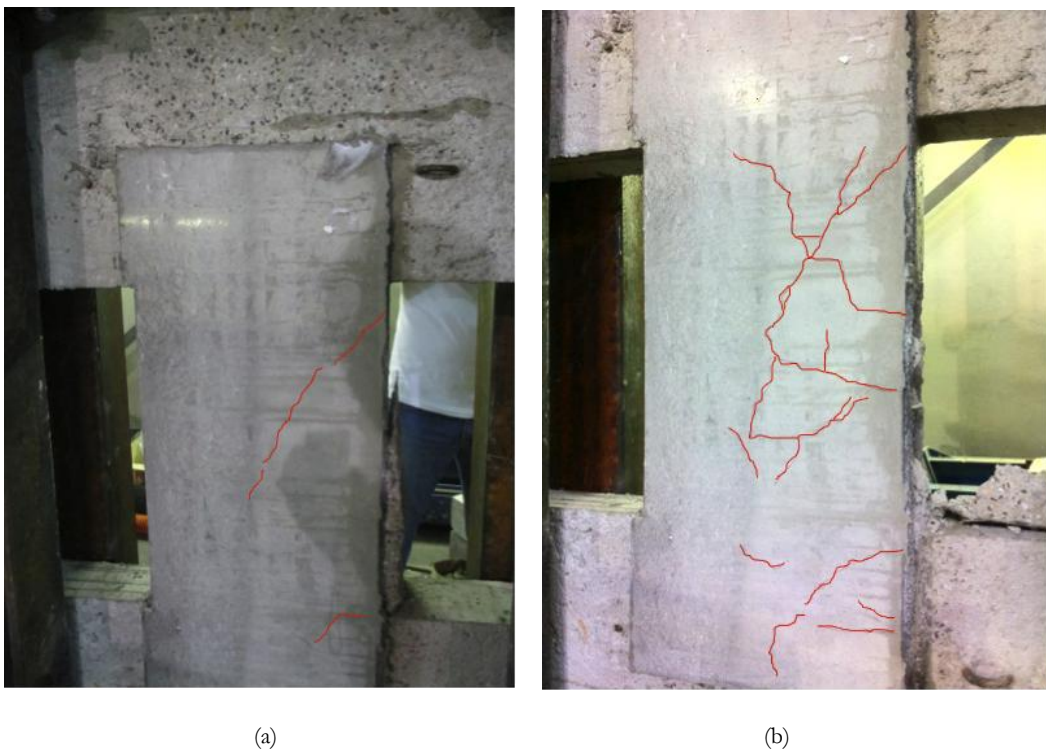
Figure 6.31 – Coupling beam repaired with HPFRCC (at 2% pre-damage level) at failure: (a) front and (b) rear
