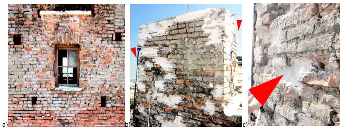
Figure 3-8 a)Walls between two openings; b),c)The degradation of bricks and repair mortar
