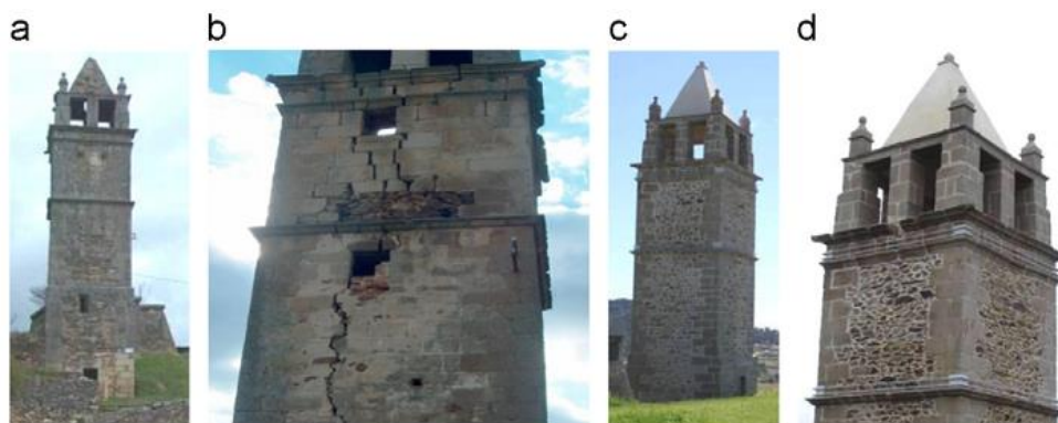
Figure 1-14 Mogadouro Clock Tower: (a,b) before; (c,d) after rehabilitation works (Ramos et al. 2010)
