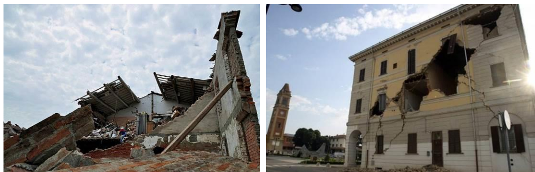
Figure 3-2 Buildings damaged by the earthquakes of the spring 2012
