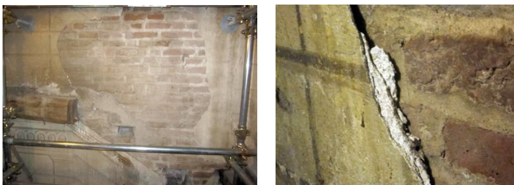
Figure 3-16 Detail of wall texture in correspondence with gaps render (about 16 m from the top). The equipment is ordered and the mortar of good consistency.
