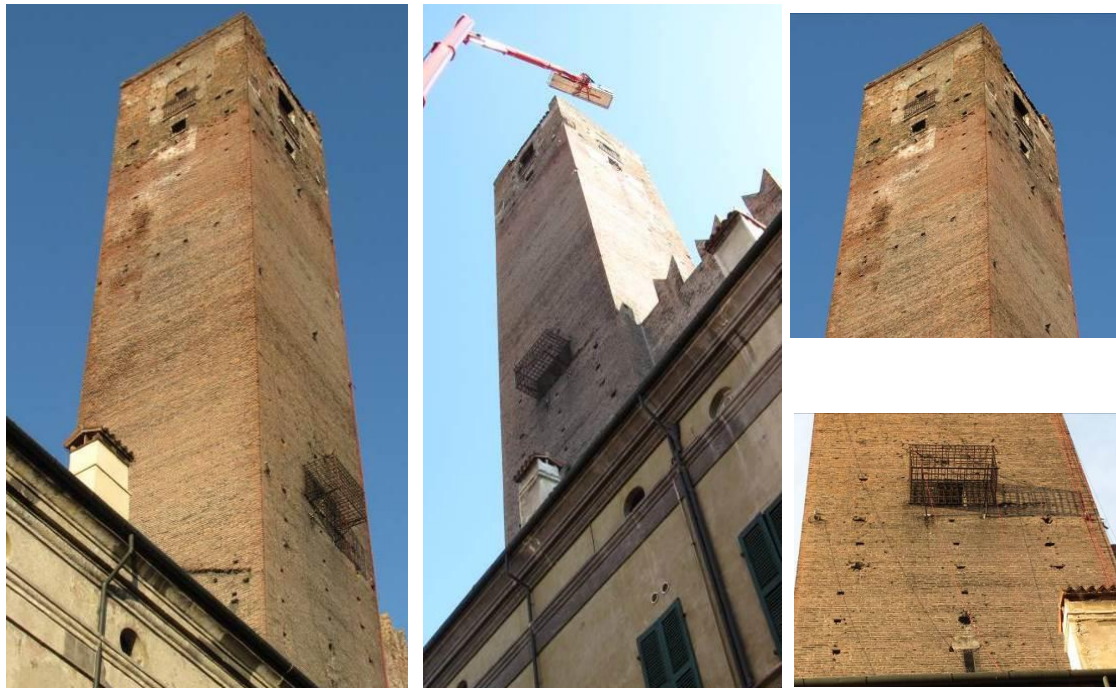
Figure 0-2 Tower of "Gabbia": overall views and details of the top and the cage
