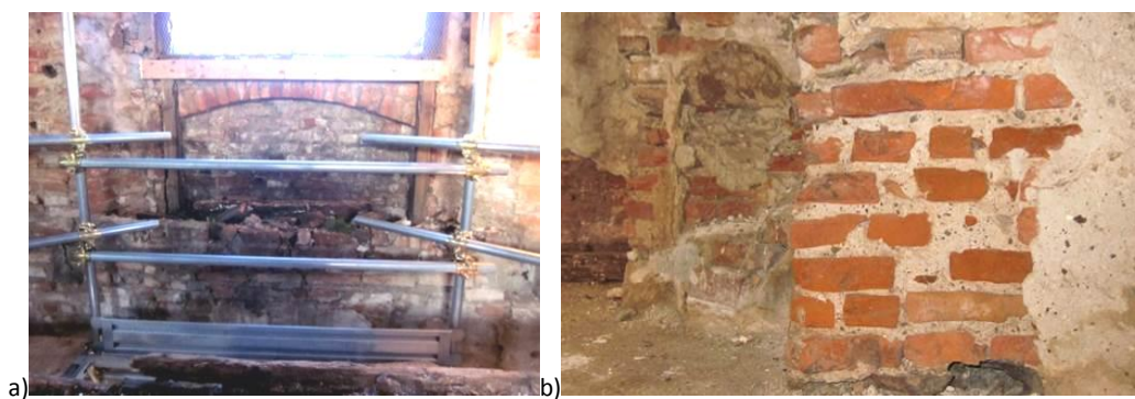
Figure 3-17 a) Detail of the opening of the interior elevation view corner Southwest and West; b) Details of the wall texture of the corner pieces to the third level
