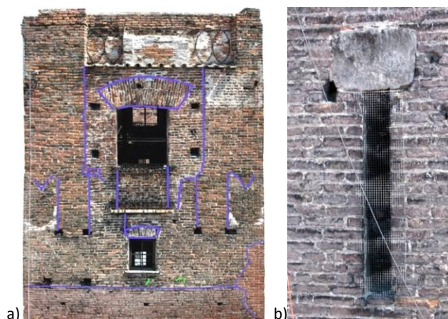
Figure 3-12 a) Top of the South-West front; b) The presence of a blocks of stone
