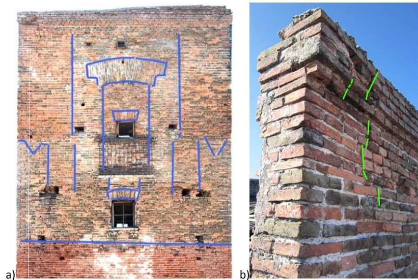
Figure 3-14 a) Top of the front North-West with highlighting structural discontinuities; b) The loss of horizontality joints and the degradation in depth of mortar joints and brick.
