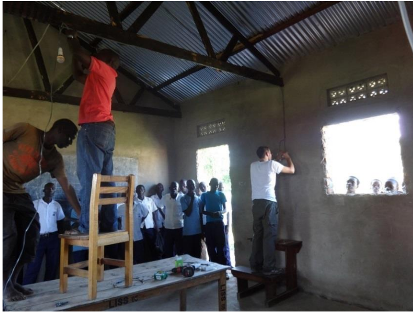
Fig 1.14 Customized system installed for Lira's secondary school in November 2013.
