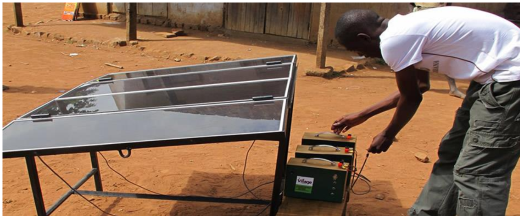
Fig 0.9 Examples of SAPV system installed by Village Energy Uganda Ltd.
