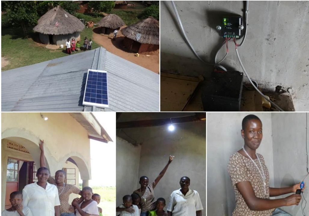
Fig 1.9 A Solar Home System (Musana 500) installed in Soroti by Village Energy Uganda Ltd.
