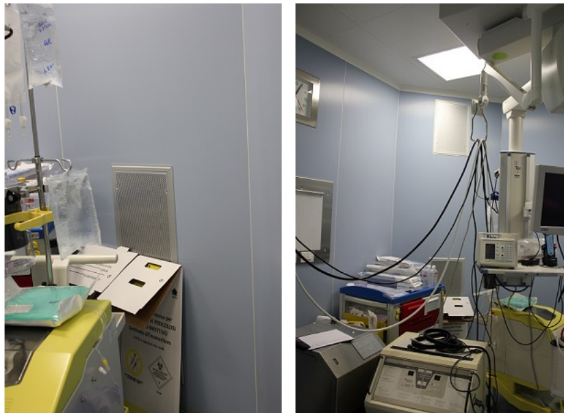
Figure 5.30: Two photo of the exhaust grilles obstructed by surgical equipment during an inspection in the studied operating theater
