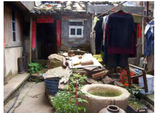
51. a dilapidated courtyard, photo credits: http://www.chinacitysearch.com/
