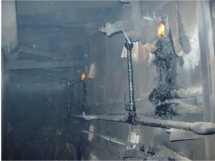
Figure 1-5 Original burners. Courtesy of DCHP
