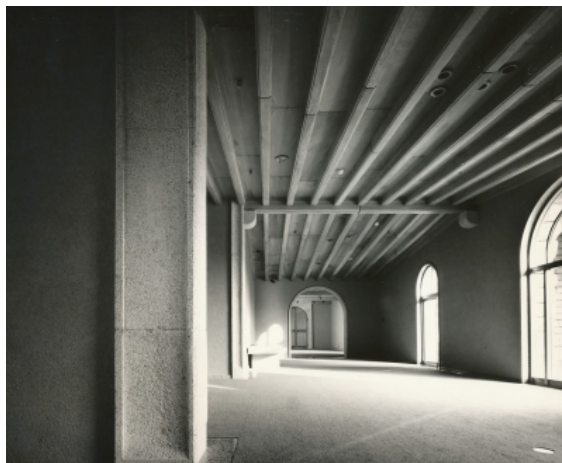
figure 2.6: Sekisuiikan (oak ceiling)
