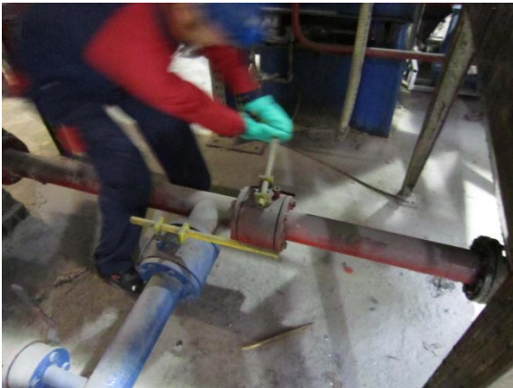
Figure 9.7 The operator is opening the valve of resin L (red tube) and the valve for the resin C is closed (blue tube)
