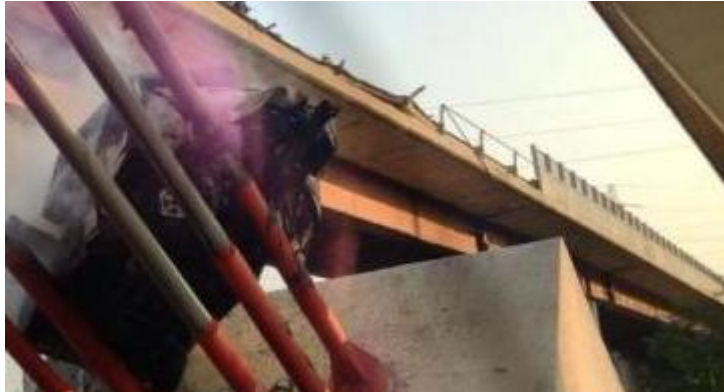
Figure 1.3. Example of accident involving bridge safety barriers (Florence, July 13 th 2013) [4].
