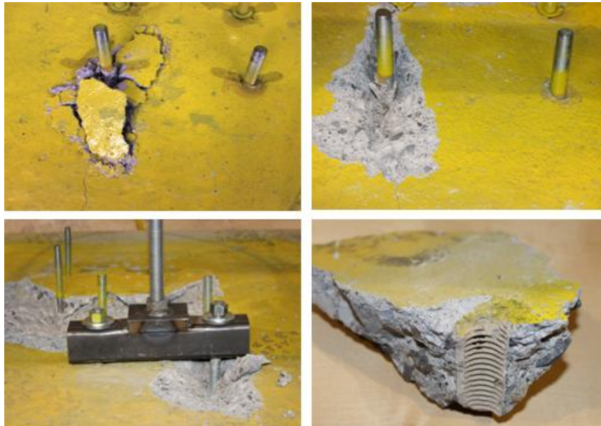
Figure 5.20. Failure mode of the anchor bolts.
