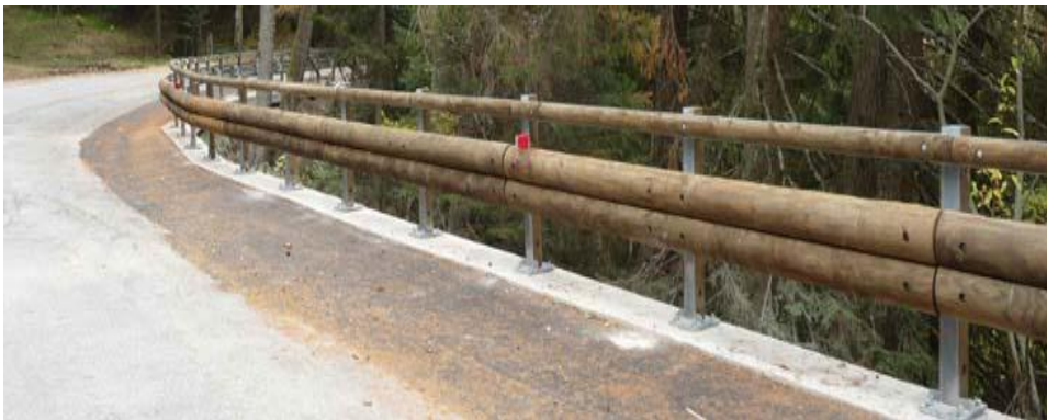
Figure 6.3. Example of wood and steel made barrier.
