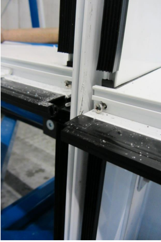
Figure 8-25: screw coming out in connection transom-mullion (after dismounting)
