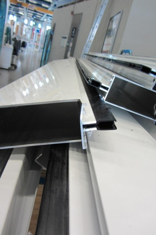
Figure 8-24: distorted transoms (after dismounting)
