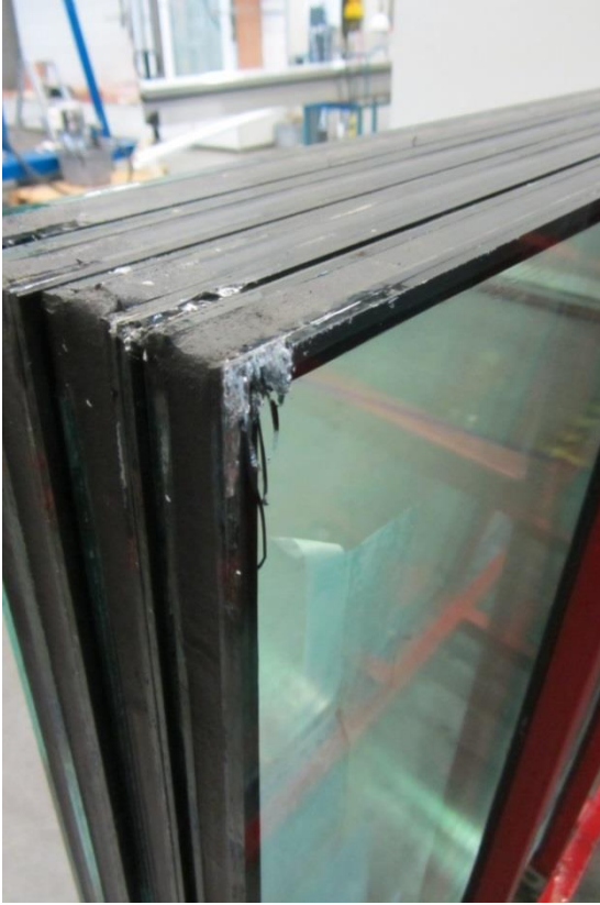
Figure 8-26: fragmented glass in the corner (after dismounting)
