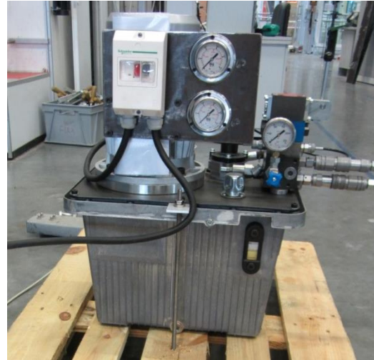
Figure 8-16: picture of the motor with the hydraulic pump
