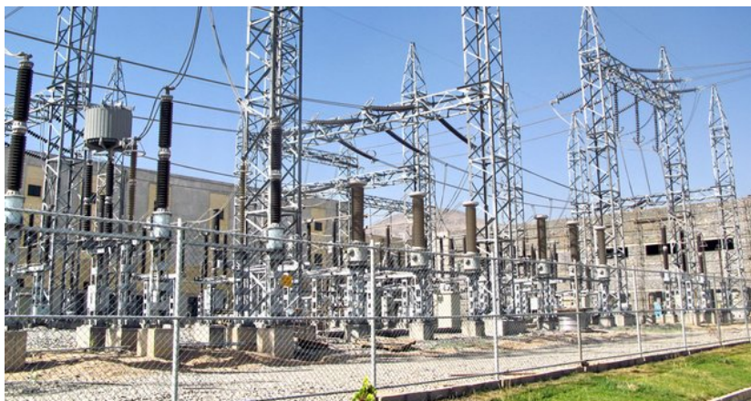
Figure 67 Power station of Company C.
