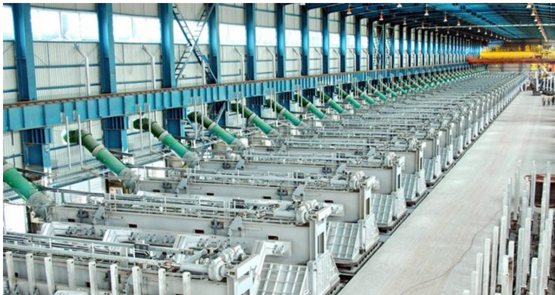
Figure 66 Pots line in new reduction cells technology, Company C.
