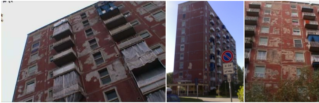
Fig 6. 4: the building condition before
