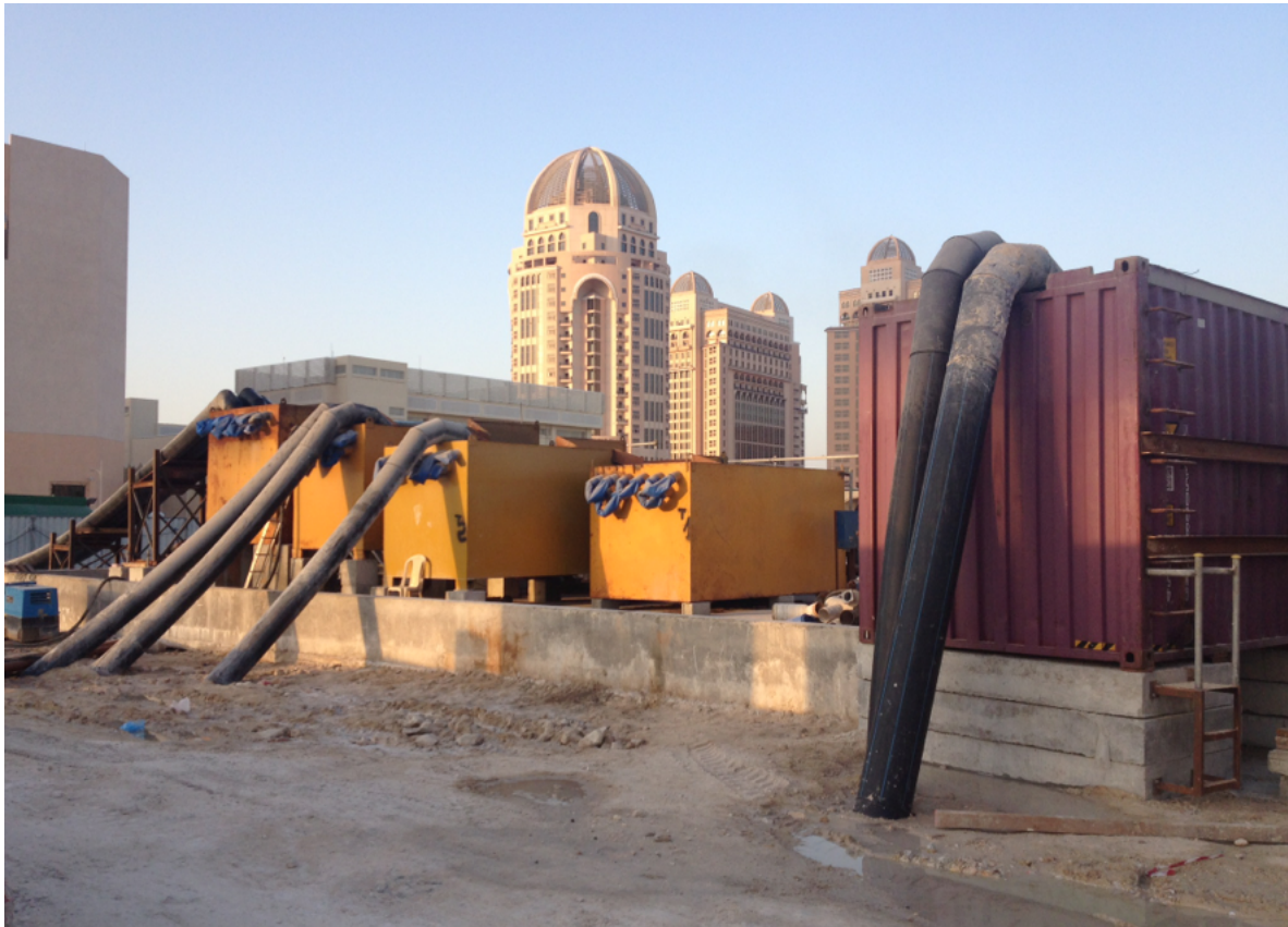
Figure 13: Final Dewatering Tanks Arrangement
