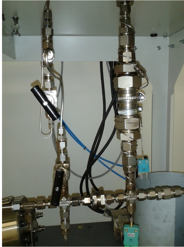
Figure 2.28. Big Reactor and Additional heating line.
