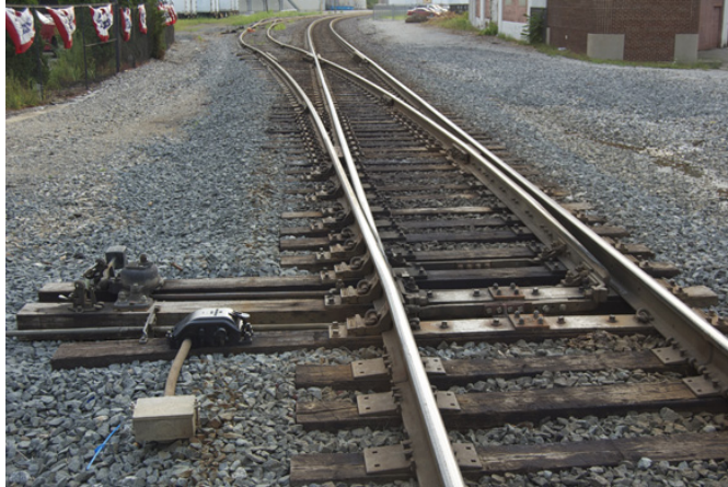
Figure 2.2: Typical example of a long turnout [4]
