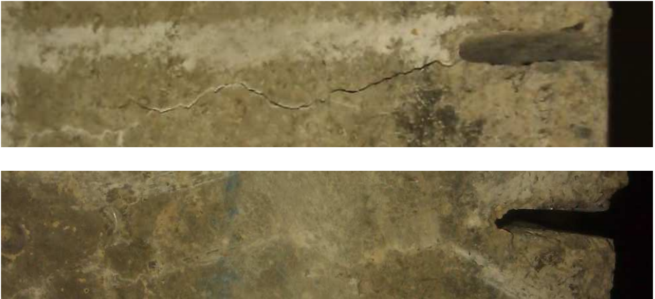
Figure 44: level of crack sealing after 30 days of conditioning for specimens precracked up to 600 \mu\text{m}
