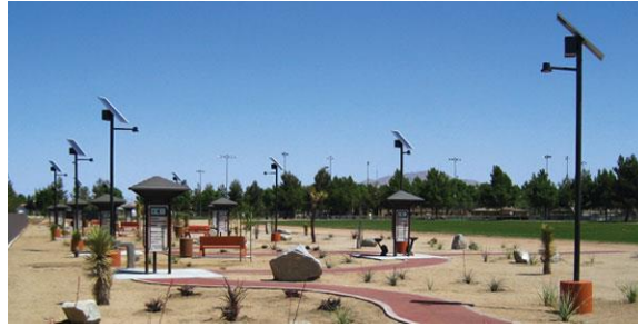
Figure 1-26: Pathway and Trail Lighting
