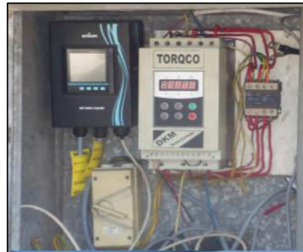
Fig. 4.22 Torque controller connected to a chiller
