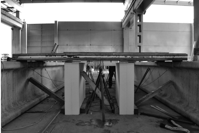
Figure 7.13: Full scale panel after the SLS test.
