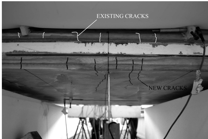
Figure 7.16: SLS full scale panel test: multi-cracking of the lower TRC face after test.
