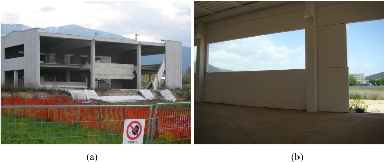
Figure 1.6 – Behaviour of cladding panels: (a) the collapse of vertical panels dragged the floor member to failure, (b) undamaged building with large permanent relative displacements among panels
