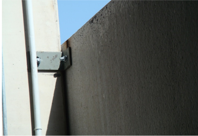
Figure 1.4 – Emergency intervention on horizontal cladding panels with several thick steel angles per panel connected with post-installed fasteners
