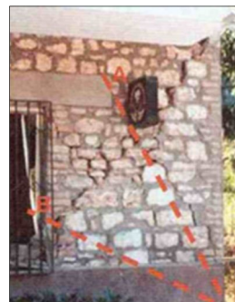
Fig 4.38: Masonry example of masonry cracks by actions coplanar with the wall (Borri, 2011).
