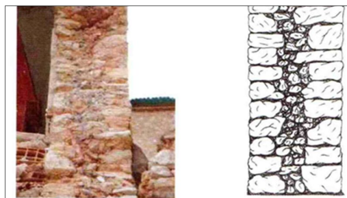
Fig 4.23: Lack of diatones inside of the masonry (Borri, 2011).
