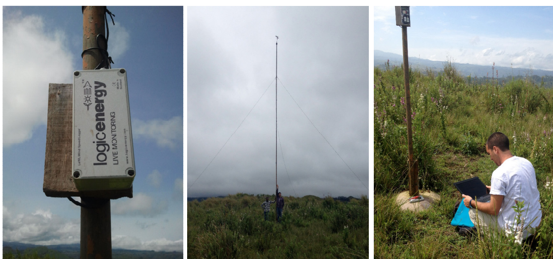
Figure 2.9 LeWL logger (left); anemometer installation (center); data acquisition (right). Source: Authors
