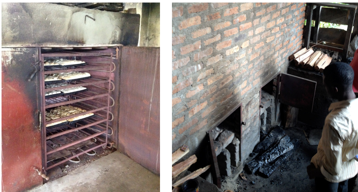
Figure 2.12 Bakery oven during operation (left); back-door for firewood inlet (right). Source: Authors
